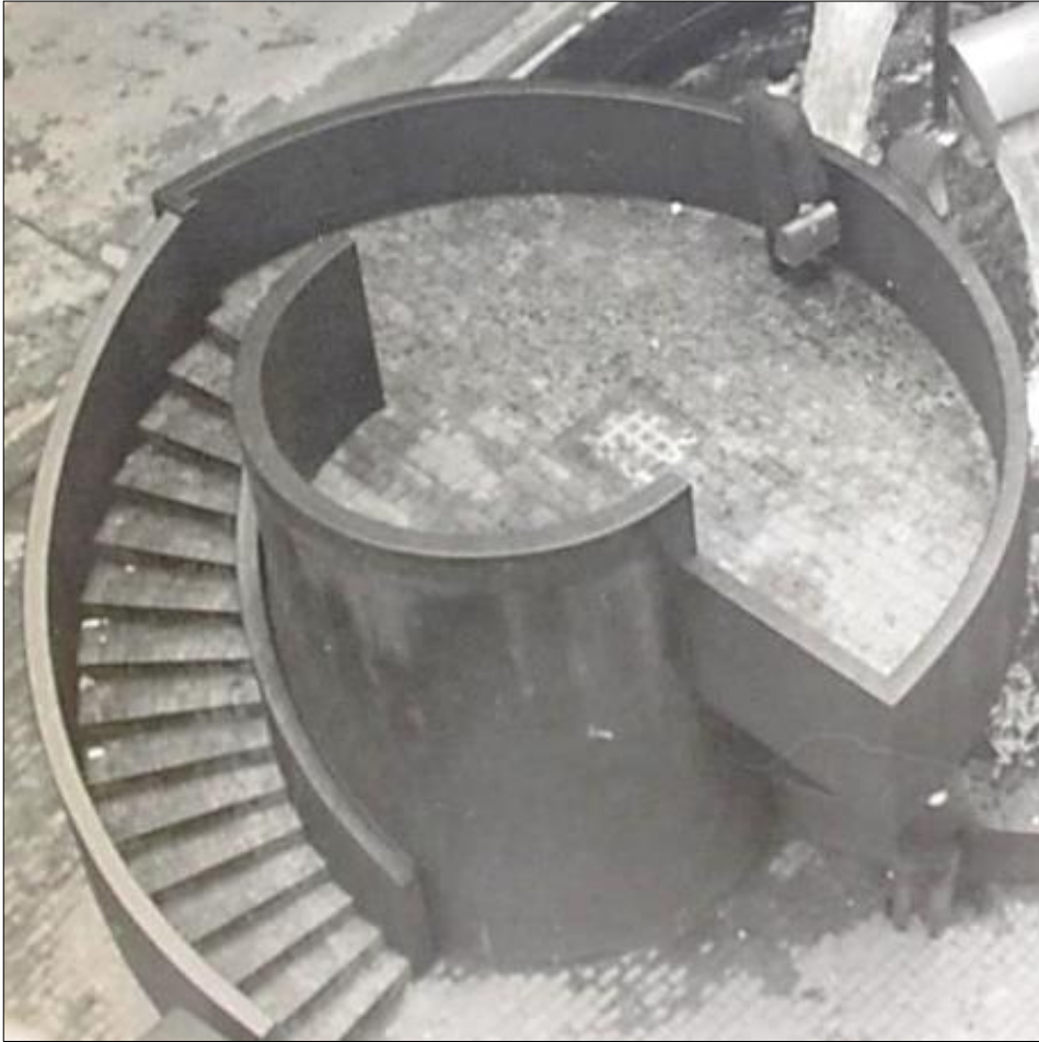
Original brindle red tiling to platforms & stairs Stairs relined with dunbar chequer plate steel
