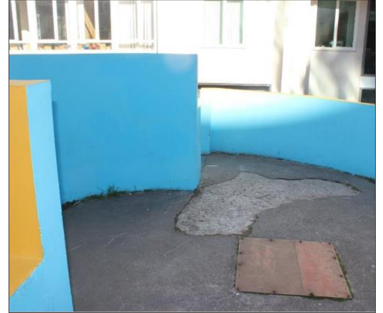
Current disintegrating asphalt floor finish to viewing platforms
