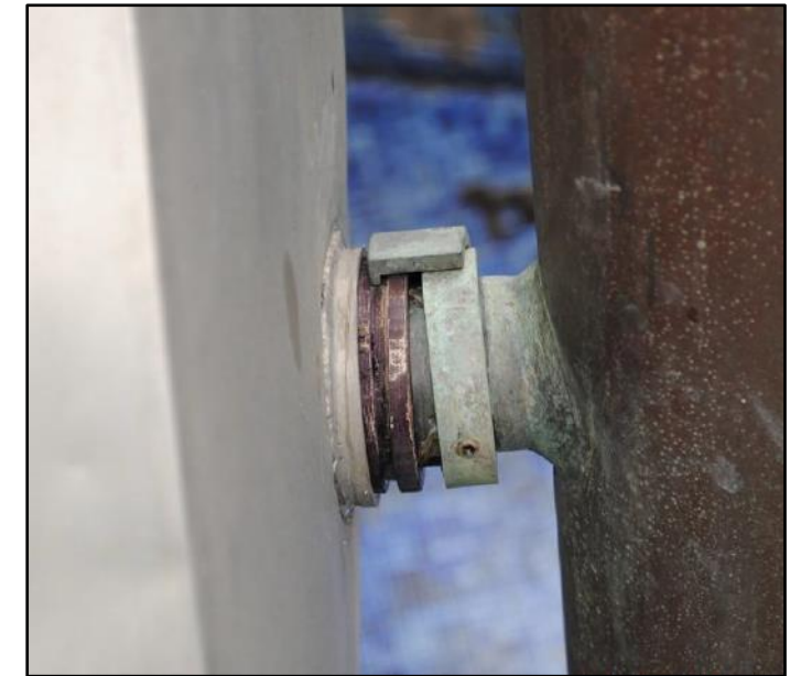
Half round fitting removed to show area from which 'buckets' leak
